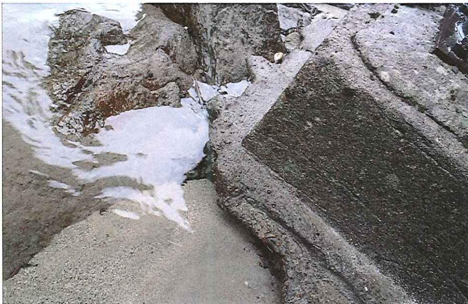
CK2395 Pier Undermining 3
